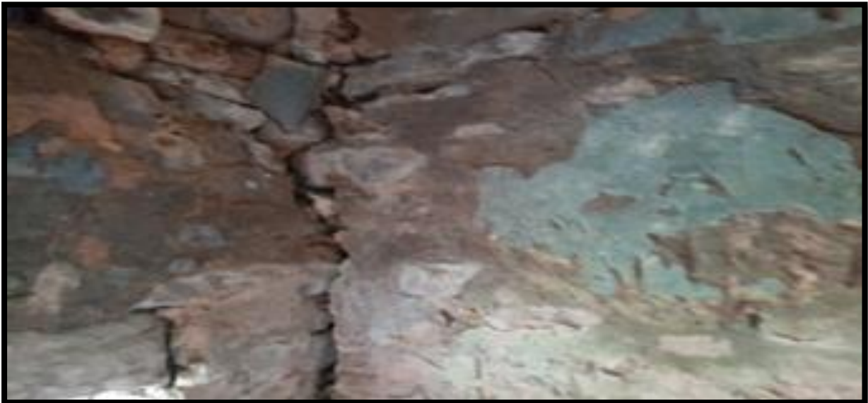
Figure 3.6 Traces of color on walls of Draid Samadhi.
