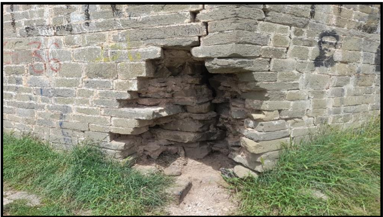
Figure 2.5 Damaged exterior wall of Gulshan-e-shauda Samadhi.
